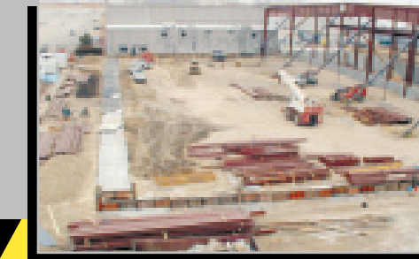
The magnitude of the project becomes more apparent as the steel superstructure begins to take shape. The steel structure should be completed by springtime. (Right)
