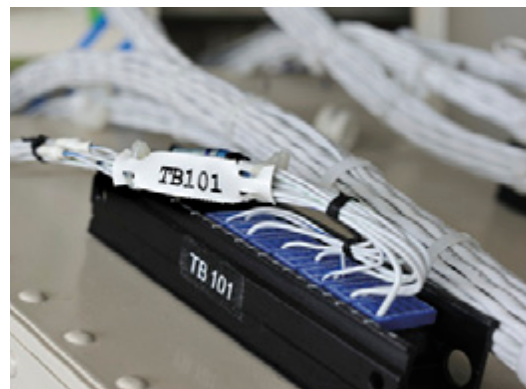
Example of our wire labeling system.
